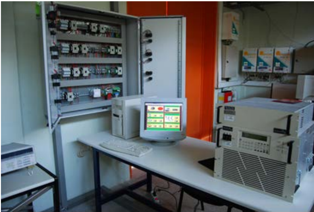
Programmable Grid simulator and load-bank control
