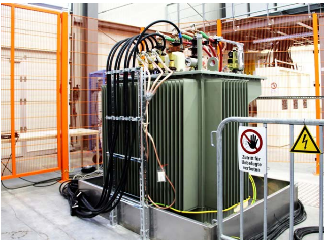
Figure 4: MV Equipment under test: Power transformer with OLTC
