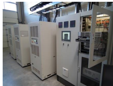
Fig. 4 Real-time system and 3 connected power amplifier (up to 270kVA) at the Fraunhofer IWES SysTec laboratory.
