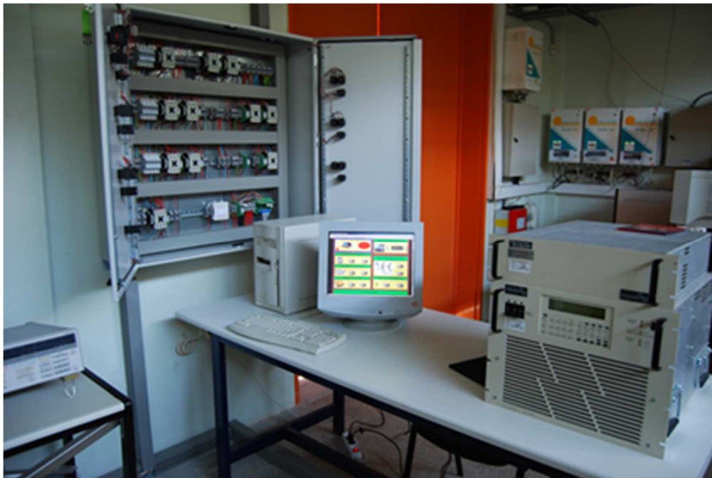
Programmable Grid simulator and load-bank control
