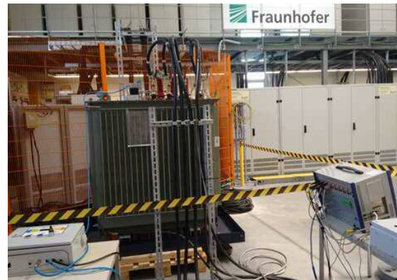
Figure 2. Smart transformer in the Test Bay
