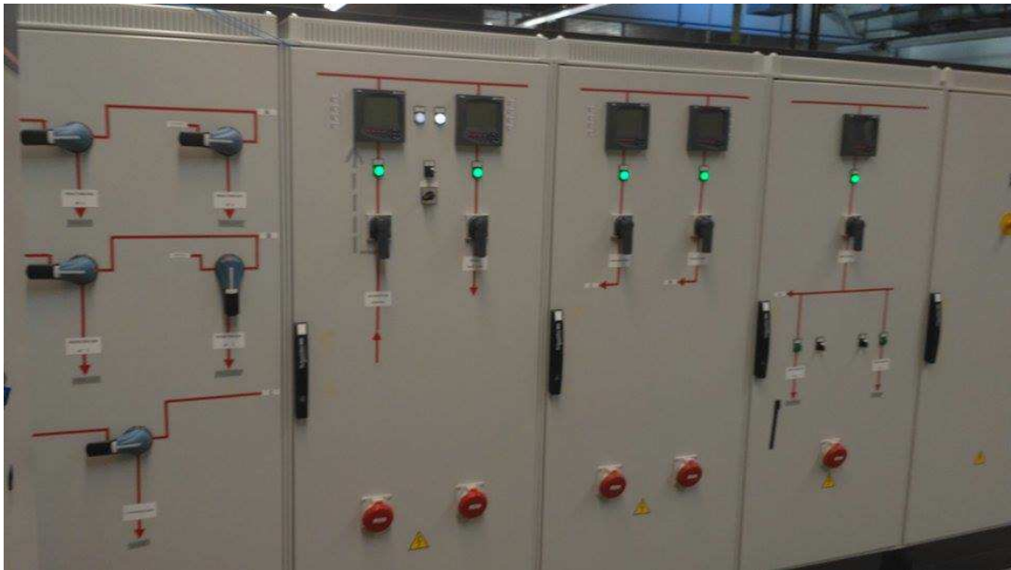
Figure 6: Grid and Inverter switches
