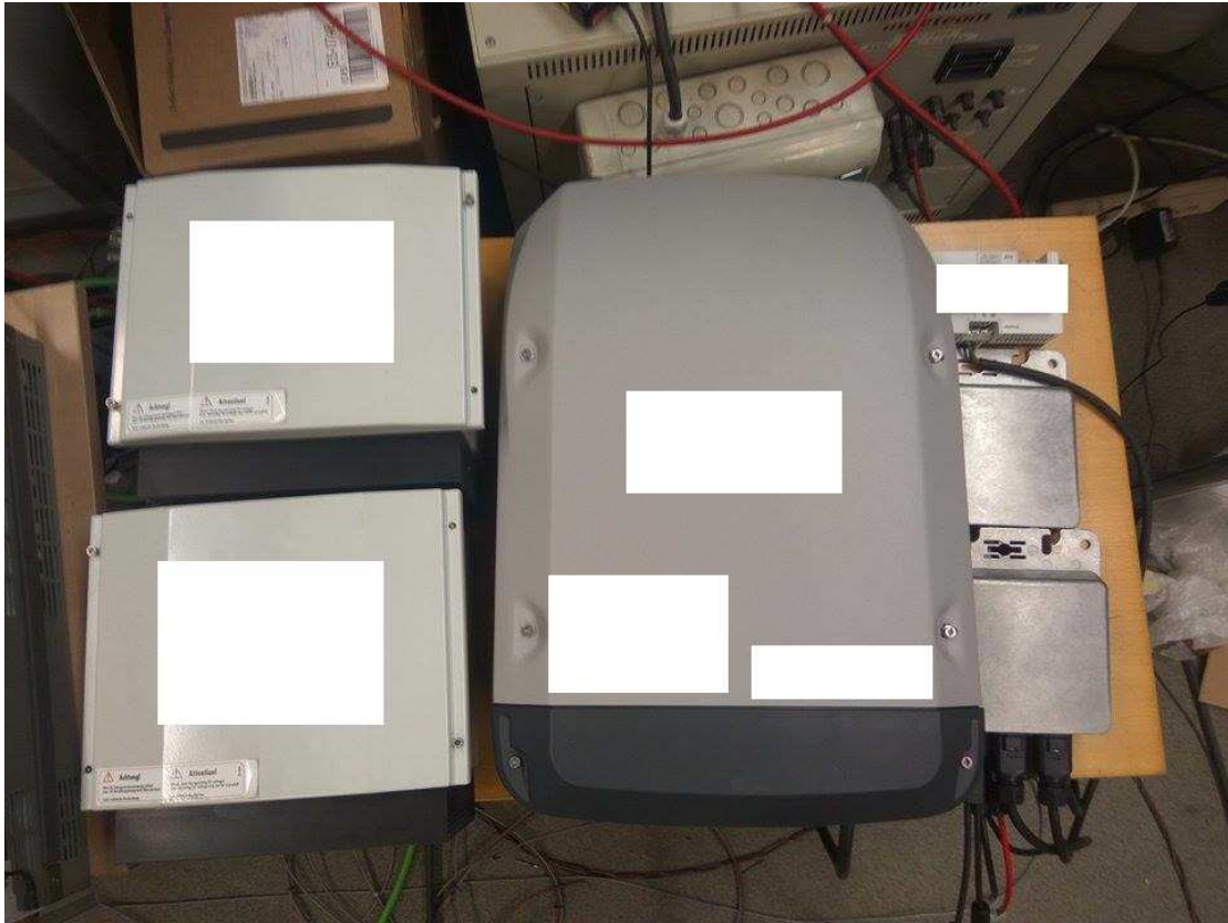
Figure 5: Inverters of the setup
