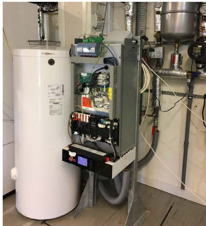
Figure 1: Picture of real heat pump Viessman Vitocal-200s Type AWB 201.B13 in DTU lab.
